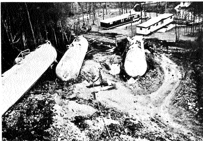
Figure 9. The 150-ft. length of welded steel pipeline built to reach the track from the pump site. Flexible ammonia hoses, 50 ft. long, with valves, were fabricated to allow unloading all three tank cars from one pump location.
