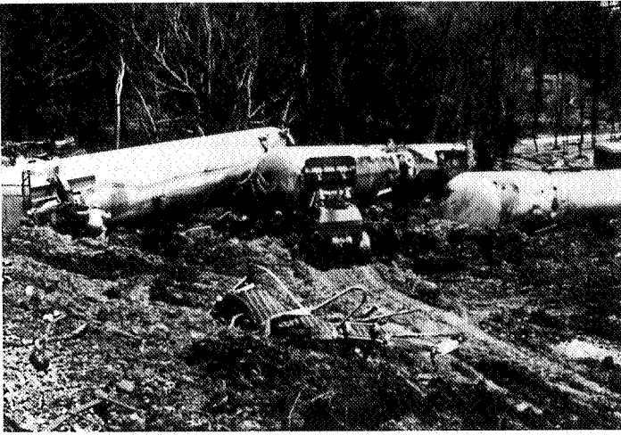
Figure 7. The loaded cars were too far away from the track to permit lifting without excessive strain on the tank shells. It was decided that a portable pump and a 150-ft. line of welded pipe would have to be built to allow transfer of contents of the three cars. All ammonia truckers had moved north with the start of the fertilizer season and thus were not available. Tanks were rolled upright for unloading.
